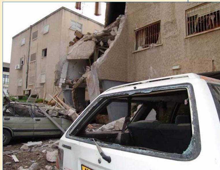
Some of the many homes and vehicles destroyed by Katyusha attacks
